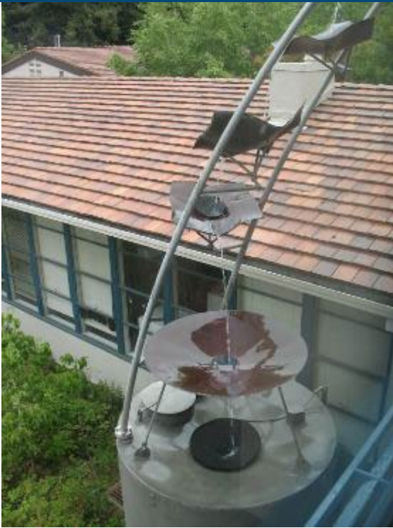
Figure 8-39 Rainwater is collected and used for flushing toilets at Mills College, Oakland.
