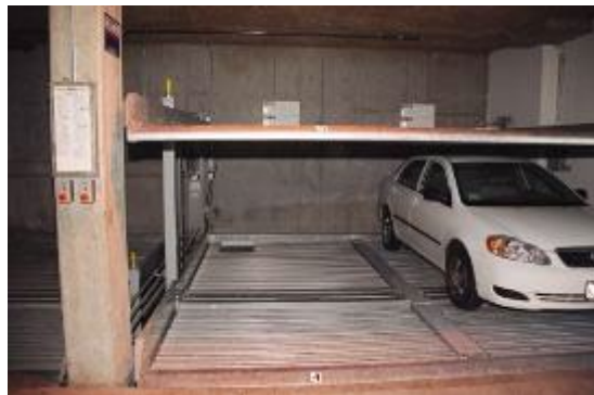
Figure 5-5. Parking Lifts in Parking Garage, Berkeley
