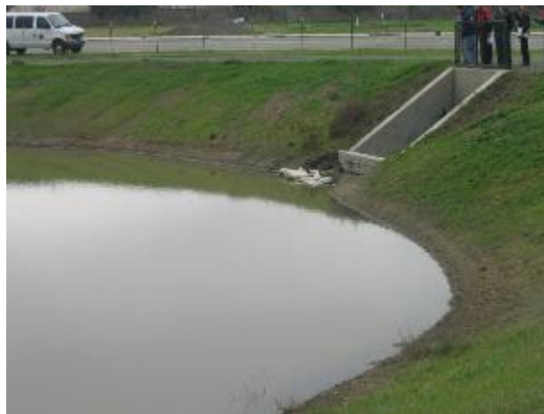
Figure 7-5 Detention pond in Pleasanton provides hydromodification management.
