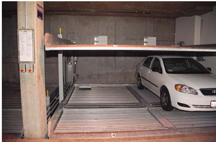
Figure 4-6: Parking Lifts in Parking Garage, Berkeley
